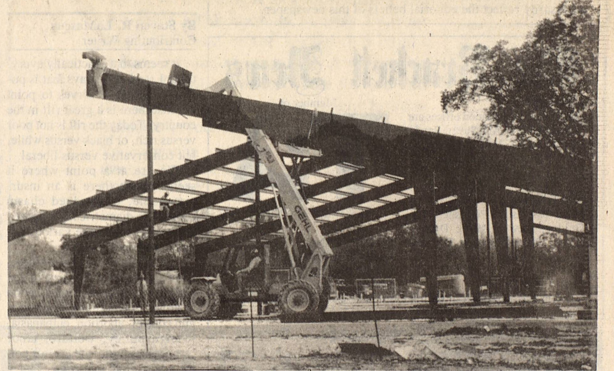
Construction crews were busy erecting a prefabricated steel framing for Brackett ISD's new high school building this week. Brackett News Photo by J.J. Guidry
