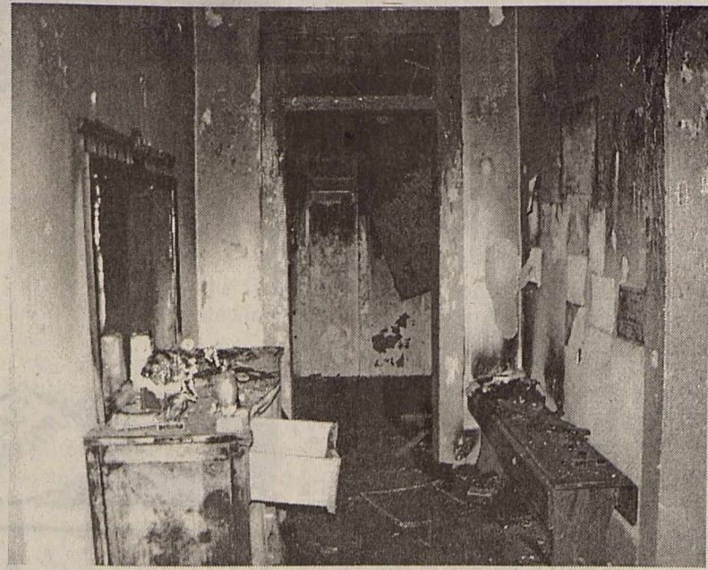
Pictured above: Inside the Resendez residence after a fire broke out Sunday morning
