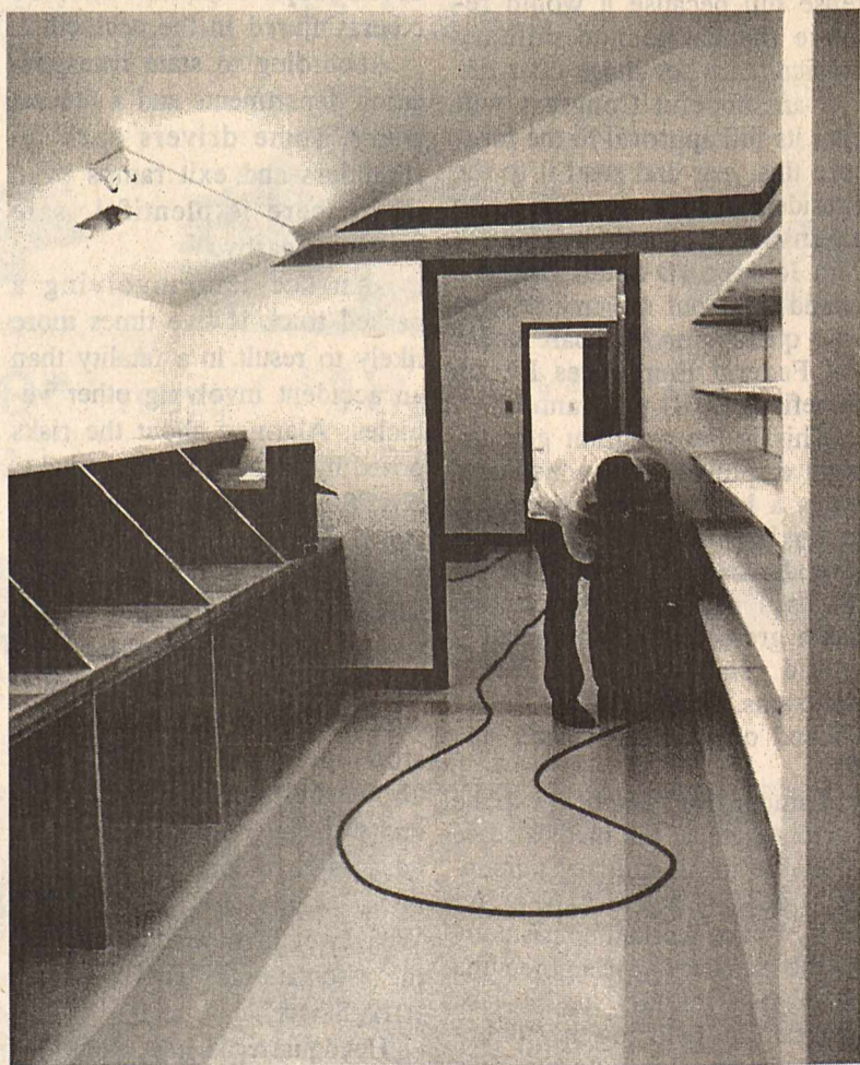
Raymond Reyes, with Jack Hill Construction Co., works on shelves in the coaches' new office. Cubicles were installed and yellow and black trimming was painted on the walls by workers.
