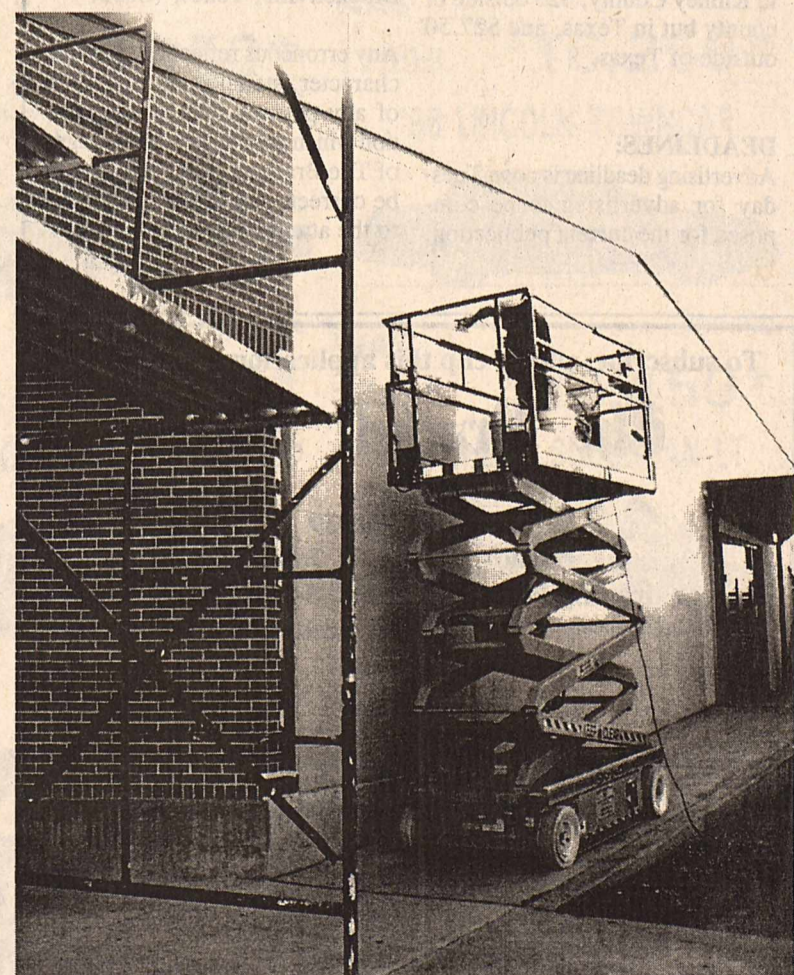
Frank Gomez paints the outside of the gym. Superintendent Taylor Stephenson said the gym and library will be painted the same color as the new building is painted - with red brick accent colors. (Photos by Diana Gonzales)
