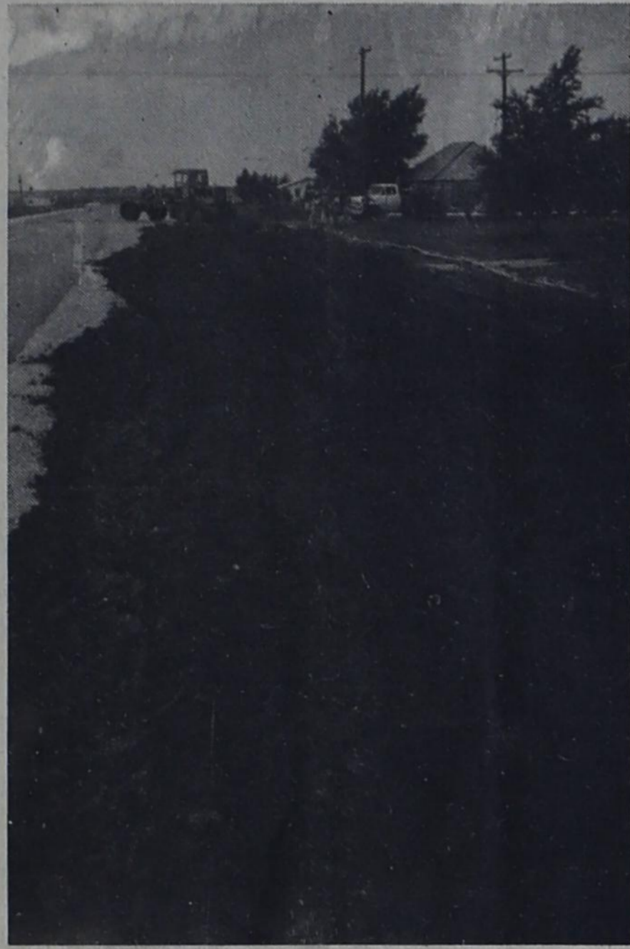
HIGHWAY 86--The maintainer in background is preparing for curb and gutter installation on Highway 86. Work shifted to Highway 86 Tuesday morning after weekend rains caused Third Street, where work was started last week, to be too wet.
