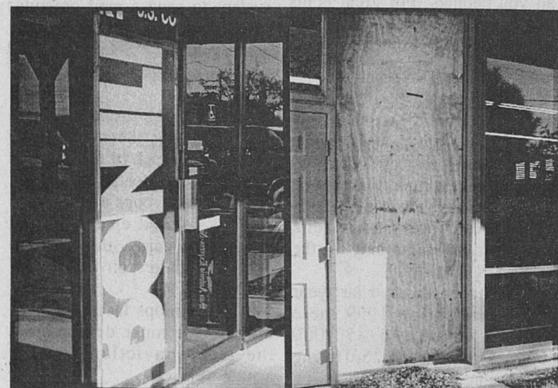
Vandals broke out glass windows at the County Library and Post Office sometime the evening of December 18th. The incident is still under investigation by the Sheriffs department.
