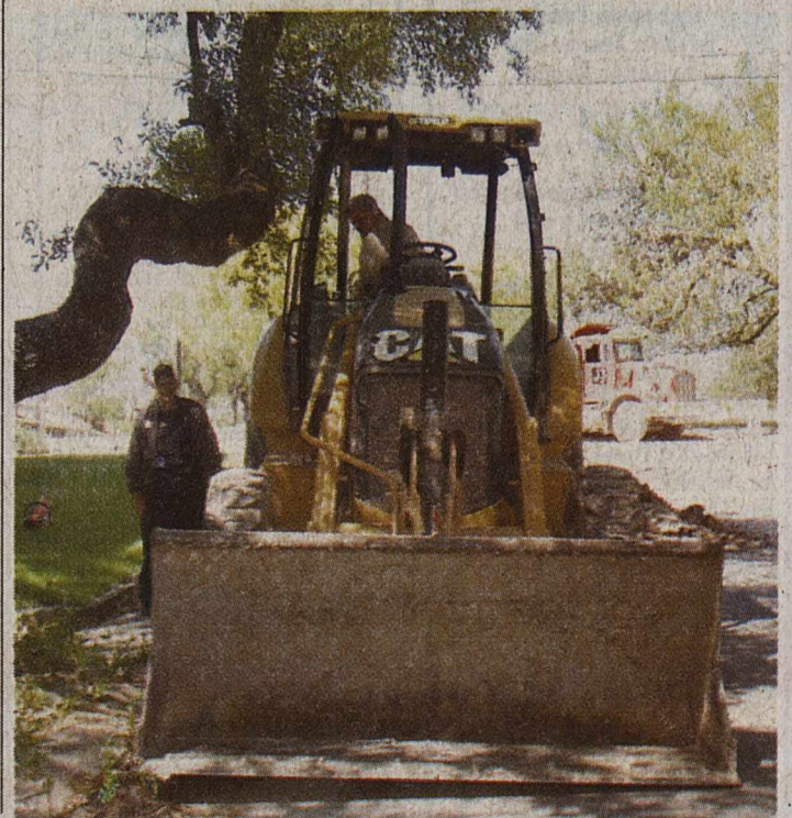
Brackett News Photo By Leigh Volcsko - From left: Fort Clark MUD General Manager Larry Sofaly and equipment operator for J3 Company Bill Simons discuss the road repairs currently underway at Fort Clark Springs.
