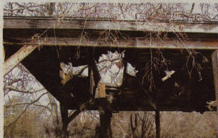
Photo Courtesy To The Brackett News - Old roof on the pergola at the newly created dog park at Fort Clark Springs
