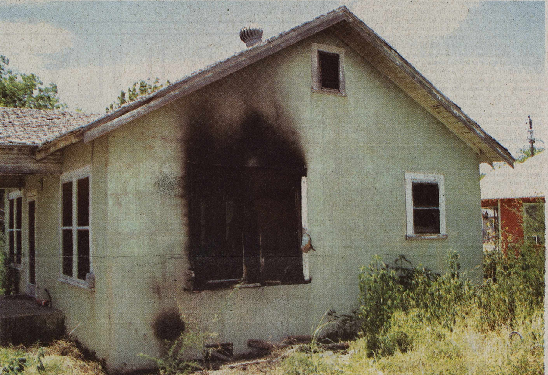
Brackett News Photo By Leigh Volcsko - A house at 501 Gove Street in Brackettville was damaged by fire early in the morning on June 23. Kinney County Appraisal District records state the home is owned by Mary LaGioia. The home was being remodeled and is among nearly a dozen homes suspected of being set ablaze by arson in the last ten years. View more photos available at mybrackettnews.com
