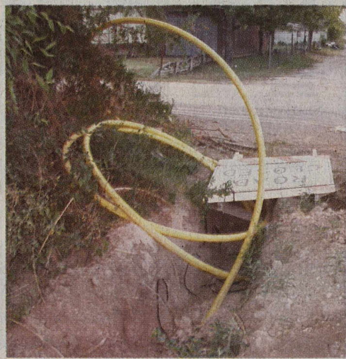
Brackett News Photo By Leigh Volcsko - New gas line being installed in the alley way between East Fulton and Veltmann streets.
