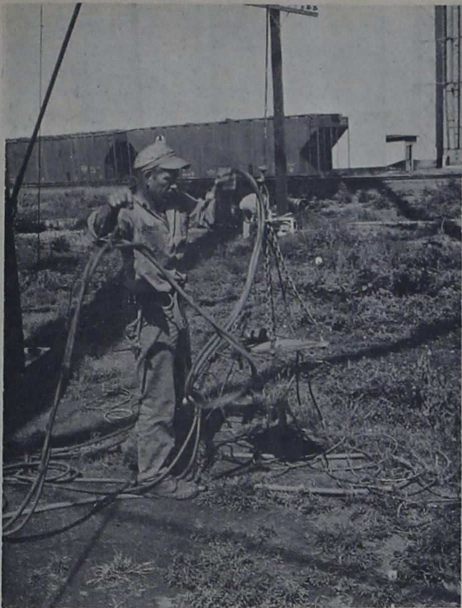
PREPARING TO ASCEND --- Although he appears to be untangling some type of mess, Eugene McFarland is actually preparing to climb onto Bovina's 100,000 capacity water tank to continue repainting work. Begun last week, the workmen have no deadline for completing the job.
