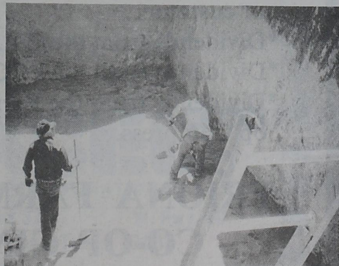
FUEL PIT... Workmen are shown putting the finishing touches on a new pit that was dug on the Charles Oil & Gas property this week to hold a huge fuel tank (see above)
