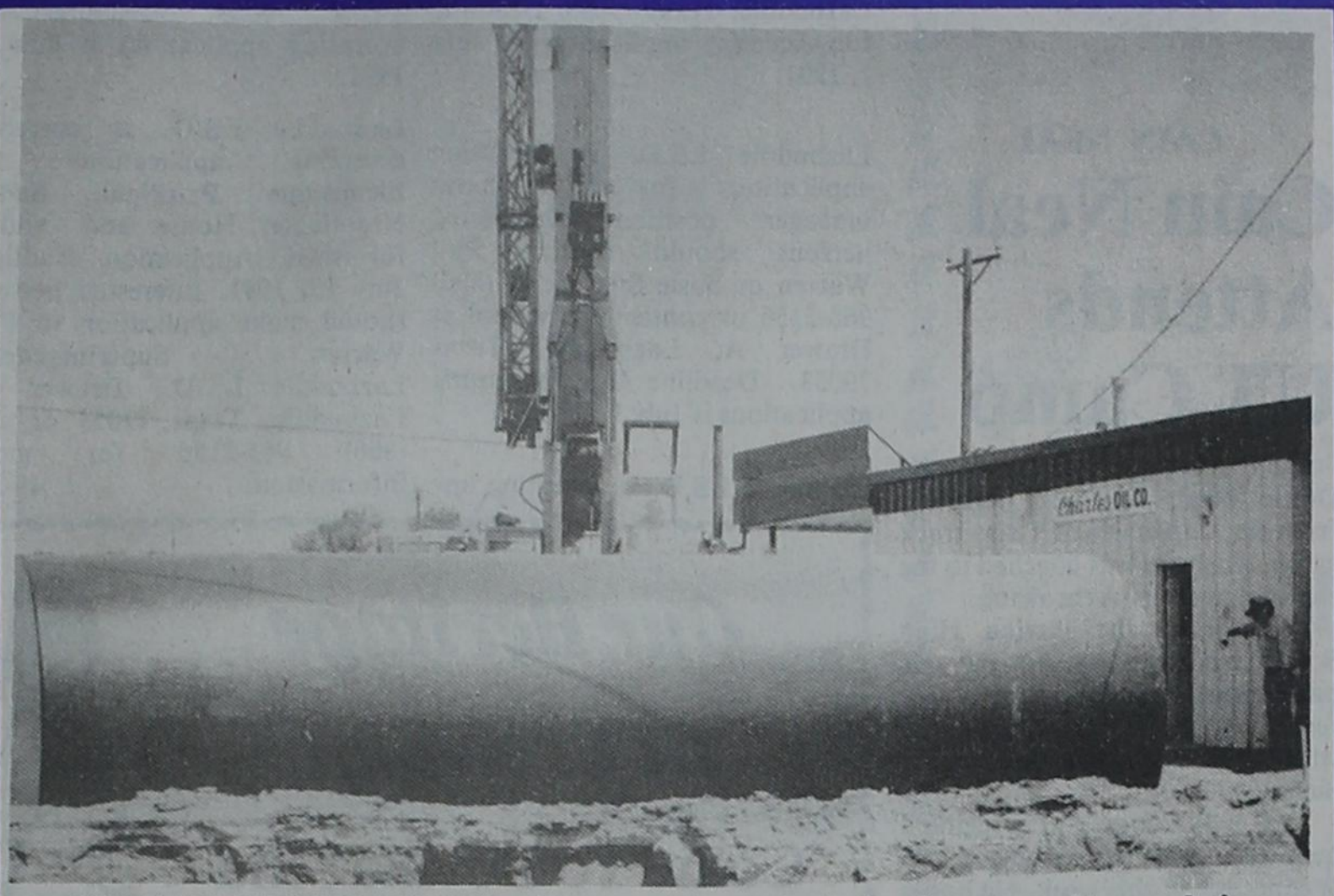
CONSTRUCTION WORK... A new storage tank is shown as it was being installed at Charles Oil & Gas Company this week. Some extensive work is underway at the local company, and a Grand Opening will be announced when all the work is completed.
