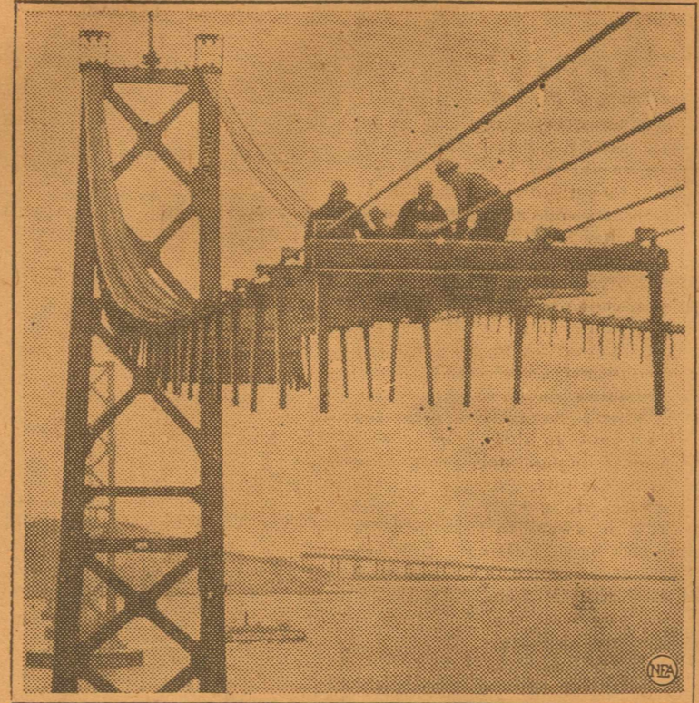
It's 450 feet down to the water, so there'd be a great chance for a grand slam with these four bridge hands—if they lost their footing. The crew is stretching the mesh flooring of the catwalk cables of the San Francisco-Oakland bridge. Approximately 71,000 miles of cable wire will be used to support the world's greatest span.
