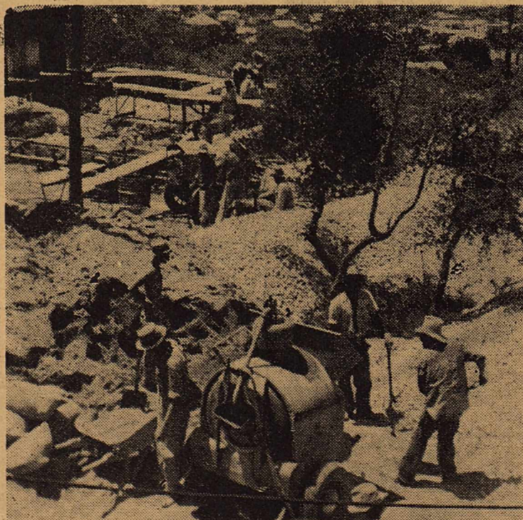
Workmen shown above are pouring foundations for the home of Sonora's new Light and Power Plant.
