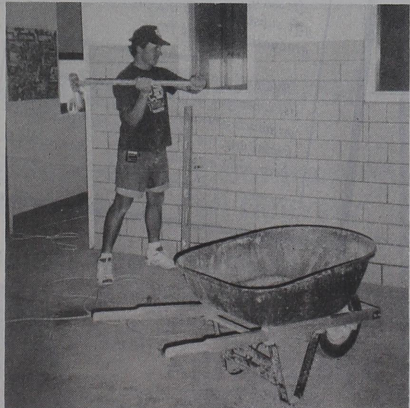
A NEW OPENING....Work continues on remodeling the cafeteria. Damian Wilhelm of Amarillo prepares to knock out a wall to prepare what will be the dish return area in the new cafeteria. Wilhelm is a carpenter and has a woodworking company that will be building the schools new cabinets.
