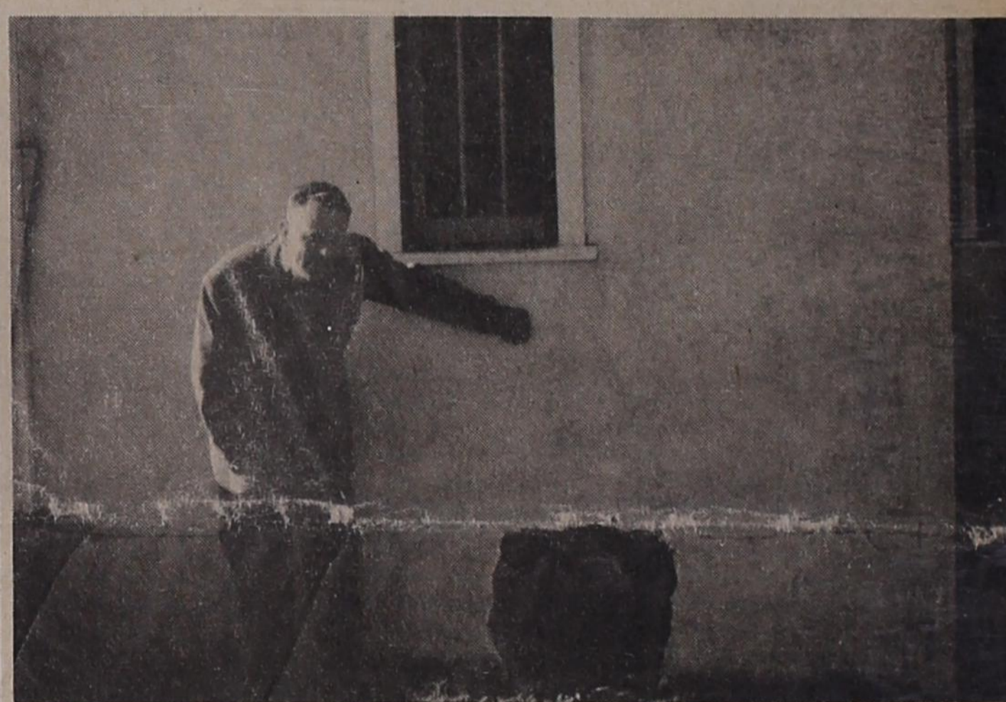
NOBODY IN THERE---Rev. John Ferguson, pastor of First Baptist Church, eyes a hole in the church building. The opening was made in preparation for the moving process that has been delayed by wet weather. Several holes such as this one have been made for men to move jacks and other equipment through when moving is started.
