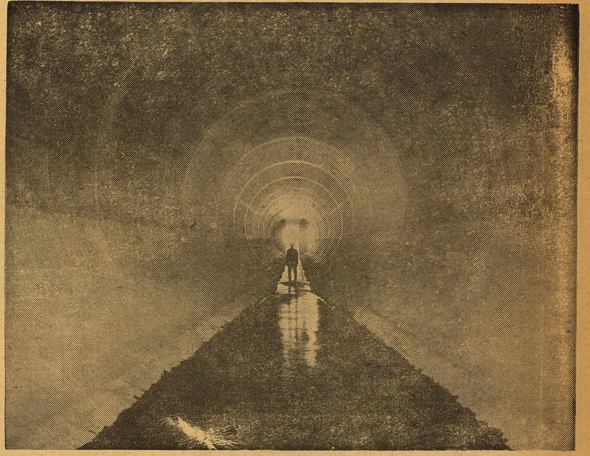
BIG TUBE —This is one of the two circular discharge conduits that will control the flow of water from behind the North Concho Dam, San Angelo's $16,200,000 flood-control project. Each of the tubes is 18 feet in diameter. Height of the six-foot workman wading through the tube gives some idea of their tremendous size. Dedication ceremonies for the dam, featuring honored guests who helped in its construction, and a tourist tour over the dam's top, will be held Sept. 16.
