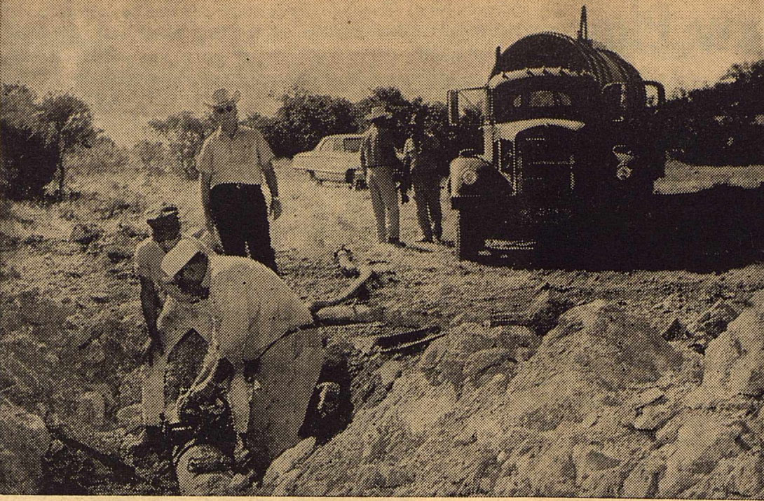
MOVING A PIPELINE was the job that these men had to do as they were working west of Sonora off the Caverns road. The new Interstate Highway 10, which is under construction, will interfere with the old Atlantic pipeline location, so a new one was laid through this rough, rocky pasture.
