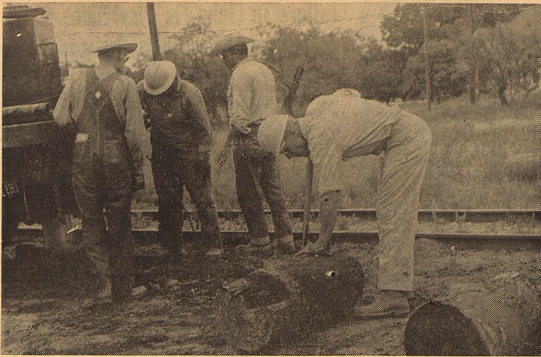
WORKMEN were in the process of clearing away some old posts and wood near the railroad tracks recently. The workmen removed the old wooden boards which ran next to the tracks near the station with the aid of a winch and truck.
