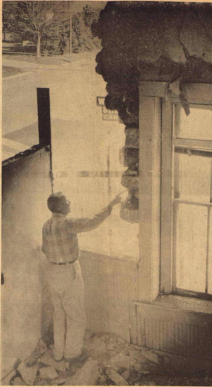
JOHN EATON POINTS TO THE REMAINING shelf of rock next to the second-story window which is perched on one large rock. The hole is in the rear of the building facing West Texas Utilities.
