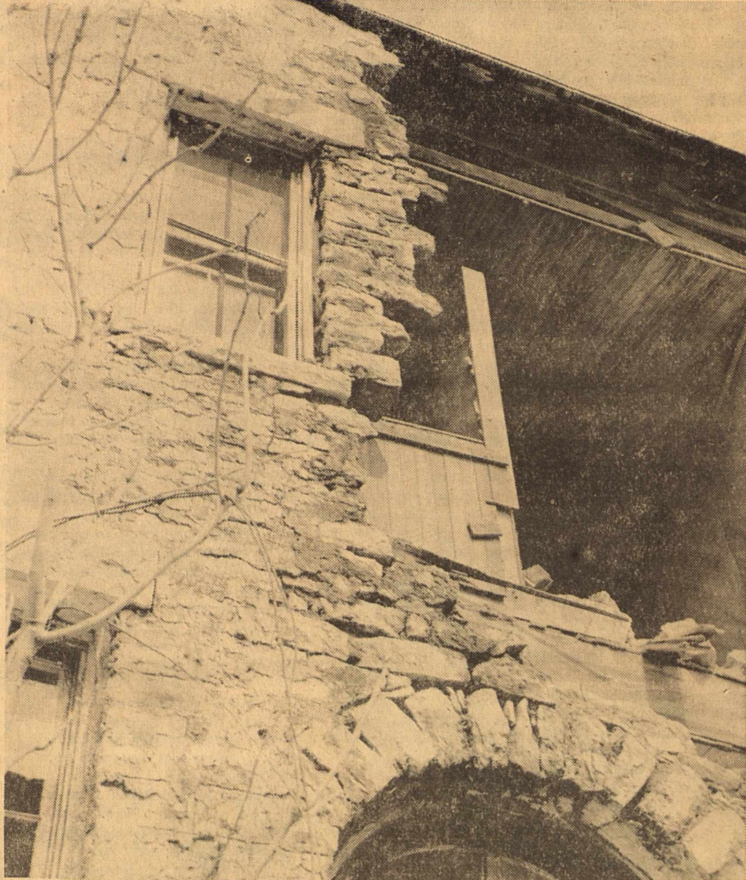
THE PRECARIOUS REMAINS of the rear of the old Mercantile Building stand at the left of the gaping hole left when the center portion of the wall collapsed Monday. Cause of the collapse is not known, but may have been caused by heavy rainfall washing the remaining mortar from between the rockwork. The building was constructed in 1902.
