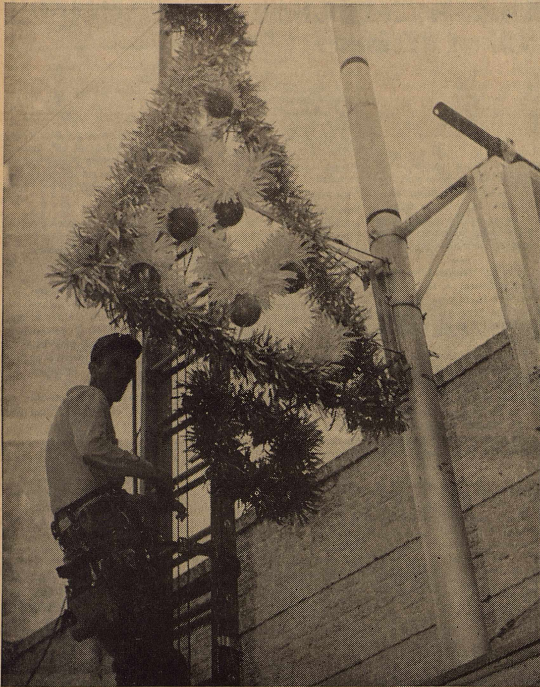
JIMMY MORGAN attaches electric wires to the new Christmas decorations being installed in the downtown area. Five decorations for poles, the Christmas tree, and tinsel crossing the intersection of Concho and Main streets make up the new decorations initially purchased. Plans have been made to add more decorations in following years.
