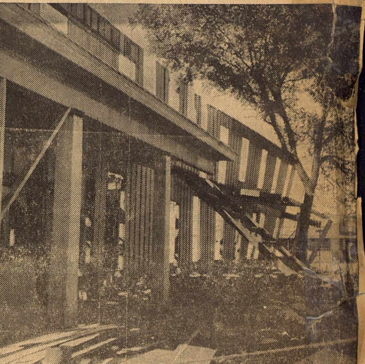
THE OLD McDONALD HOTEL is shown here in a series of pictures taken during several stages of the destruction. The roof was the first to go, then the inside walls and doors were removed. Note the 1x12's extend all the way to the top of the structure.
