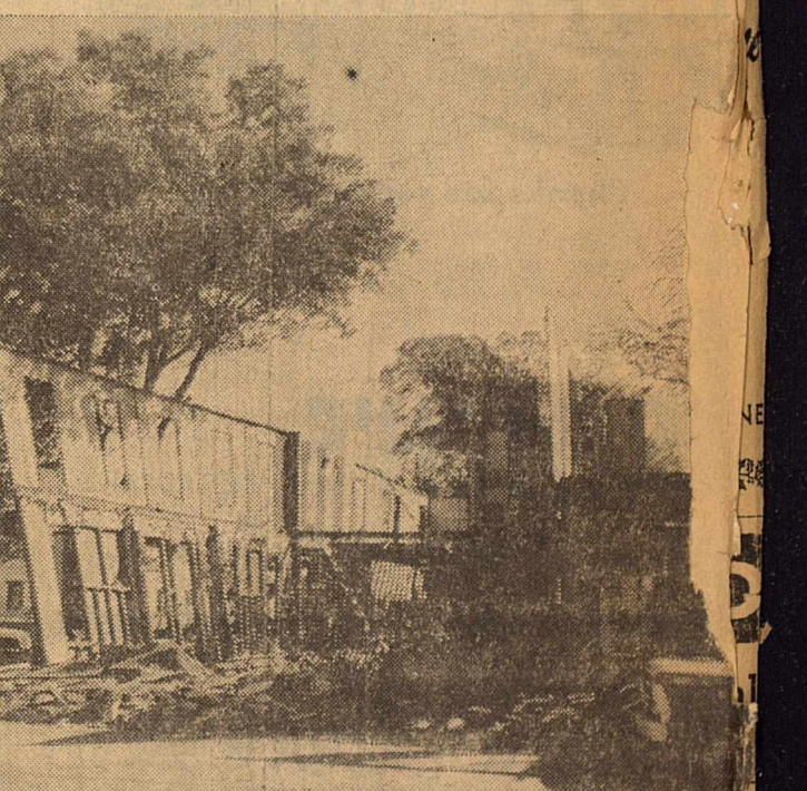
LEANING against one of the large pecan trees on the site, this wall takes a short rest before being torn down. It served the hotel for over 50 years.
