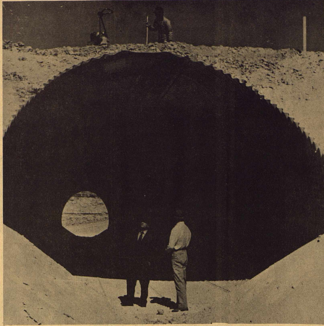
PROGRESS ON A SECTION OF IH 10 east of Sonora is clipping along at a rapid pace. Robert McCulloch, supervising resident engineer spends much of his time checking the construction. This large culvert which McCulloch (right) and J. A. Snell (left) are inspecting was placed several weeks ago. Once completed, large trucks and cattle will be able to cross through it under the highway.
