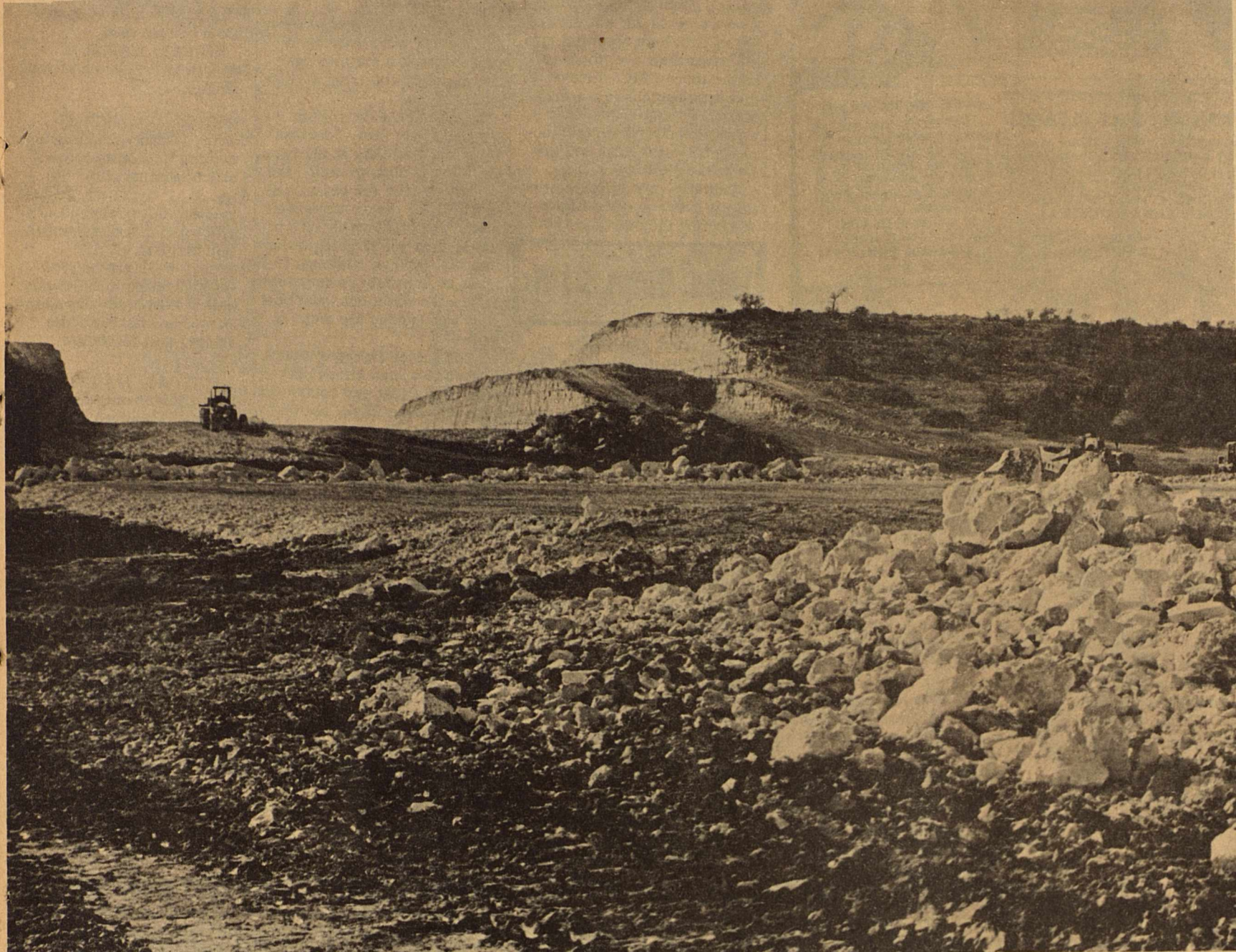
THE HILL THAT MOST SONORANS HAVE been looking at for a long time is fast changing its face as work progresses on this section of Interstate 10. Bridges are under construction and with the mild winter in this area, work on the interchange has proceeded without interruption. With two road crews and the pipeline construction crew all working here presently, the cafes and other businesses have enjoyed an unusually busy winter and early spring.
