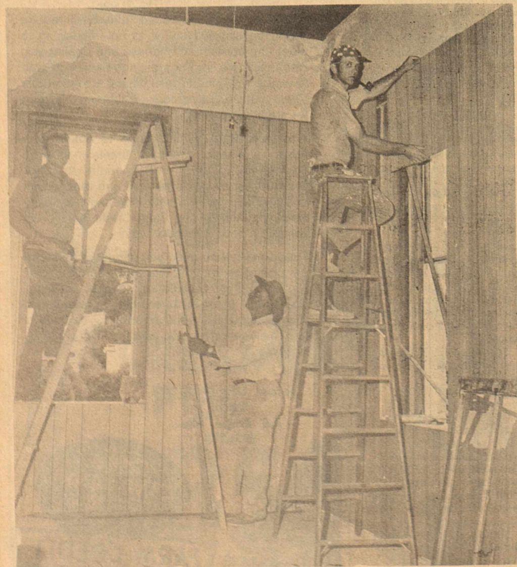
WORKMEN ARE POUNDING AWAY as progress continues on the renovation of the Junior High School building. Renovation of the building, deemed necessary to accommodate the increasing
