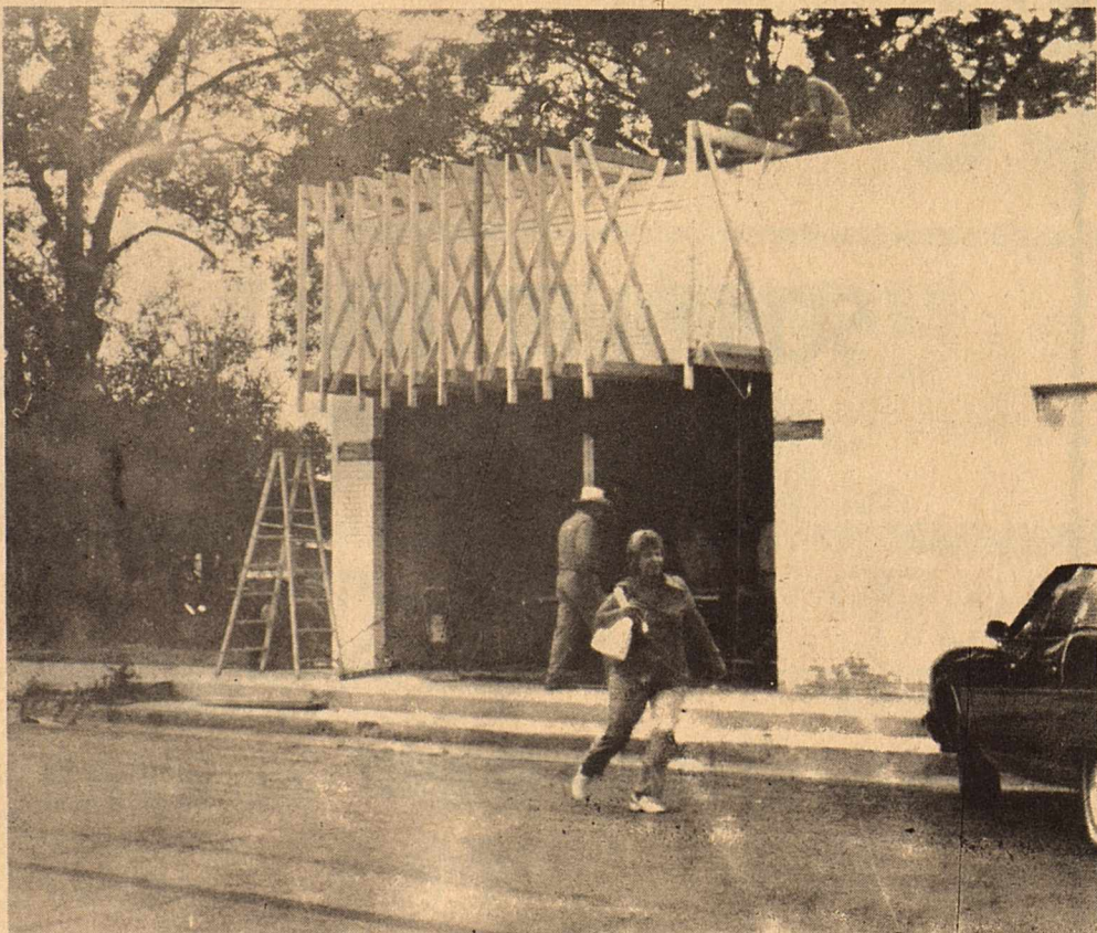
Construction began last week on the location that will house the new San Angelo Savings Association's Sonora branch office. The new savings and loan firm will occupy the building that for many years was the office of the late Dr. J.F. Howell. Approval to open the Sonora branch office was received June 26 and
