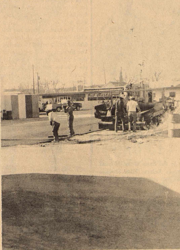
The Gulf Restaurant got a paving job this past week on their parking lot. Many improvements are being made on various businesses around town, which improves the look of the entire City of Sonora.
