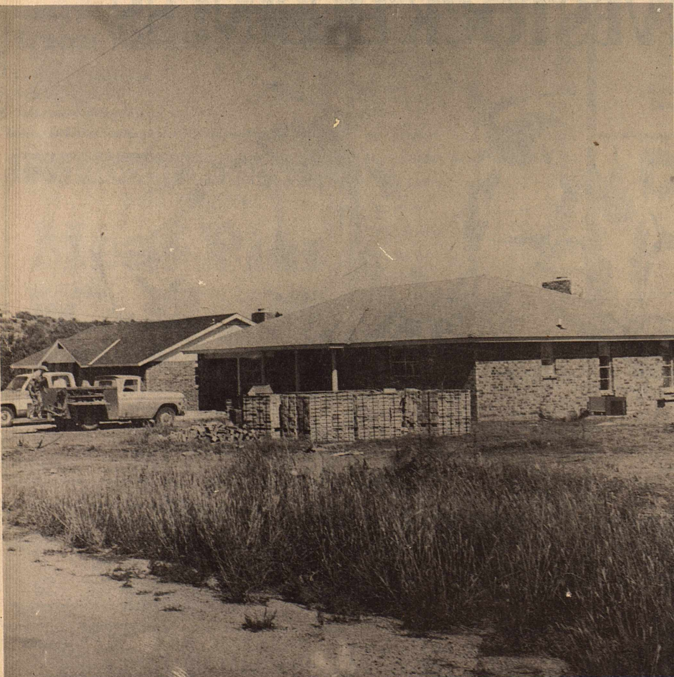
Sonora's new housing development....Meadowcreek....is beginning to show signs of growth with the construction of two new homes underway and foundation being laid for the
