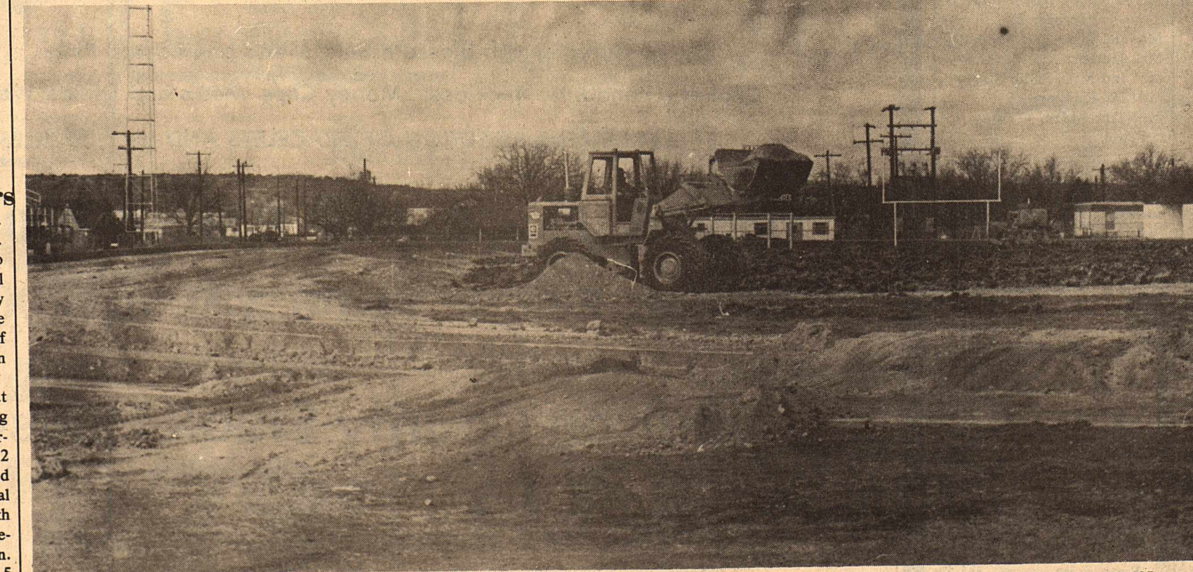
Work at the football field is progressing. Bleachers and light standards have been moved and curb work for the all-weather track is nearing
