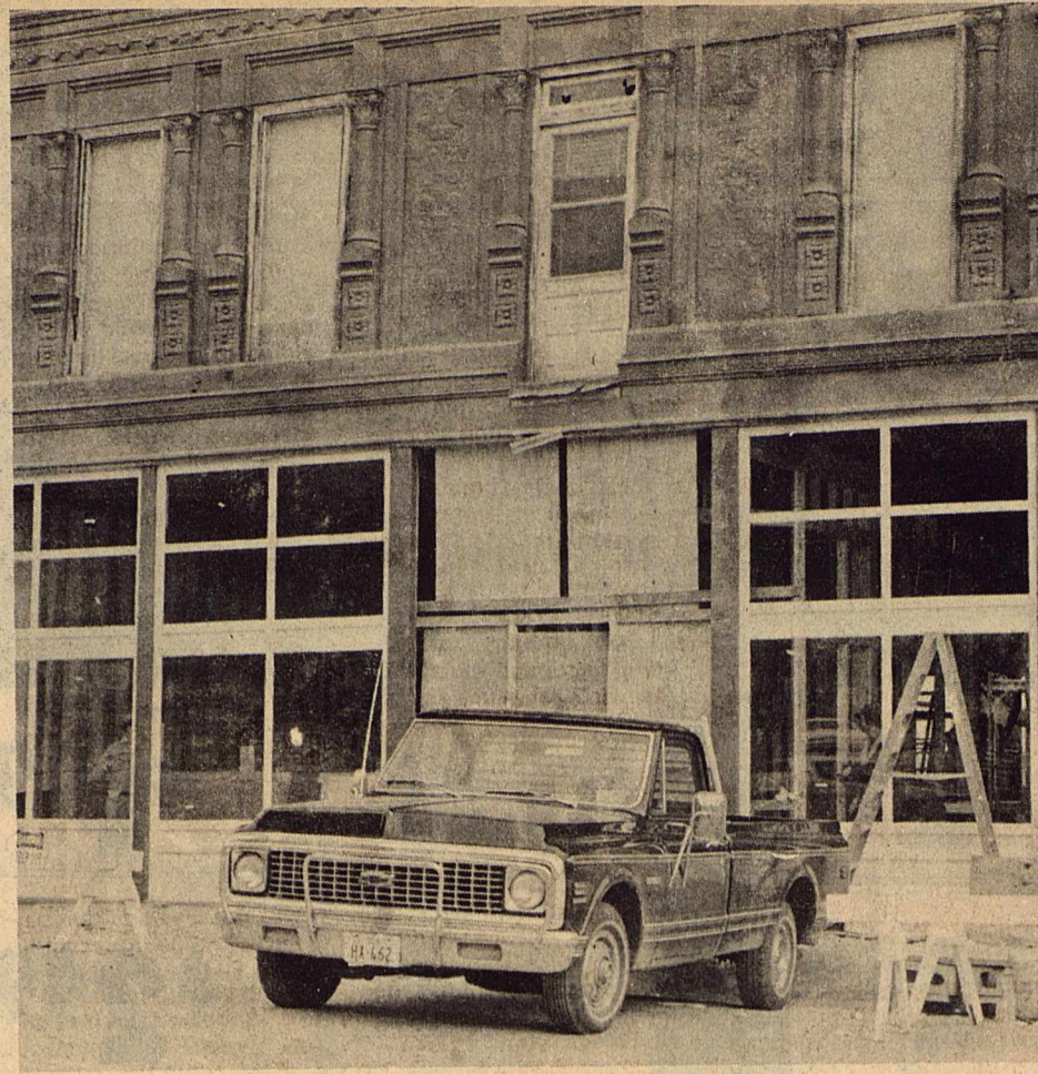
Final touches on the outside of the old Mercantile Building downtown began last week. Owner Walter Pope expects final completion for the building to be late next month.
