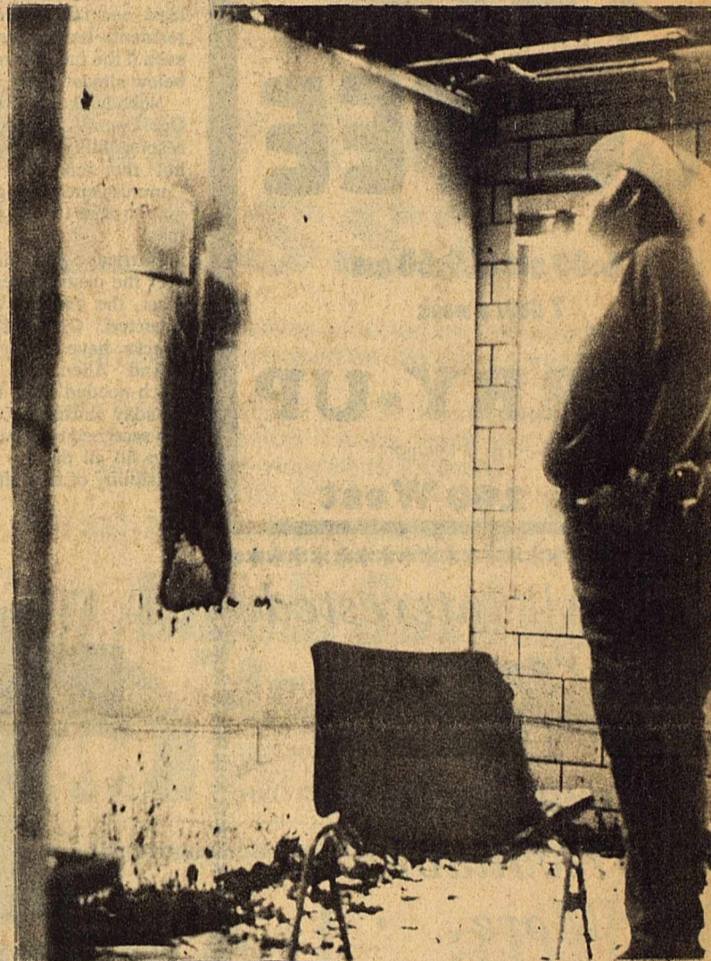
Police Chief Brent Gesch inspects the damage done by a fire at the Sonora Police Station early Friday morning. Sgt. Bill Ware discovered the fire around 1:45 am and prompt response by the Fire Department confined the fire to only one office. Gesch stated no documents or records were destroyed by the fire.
