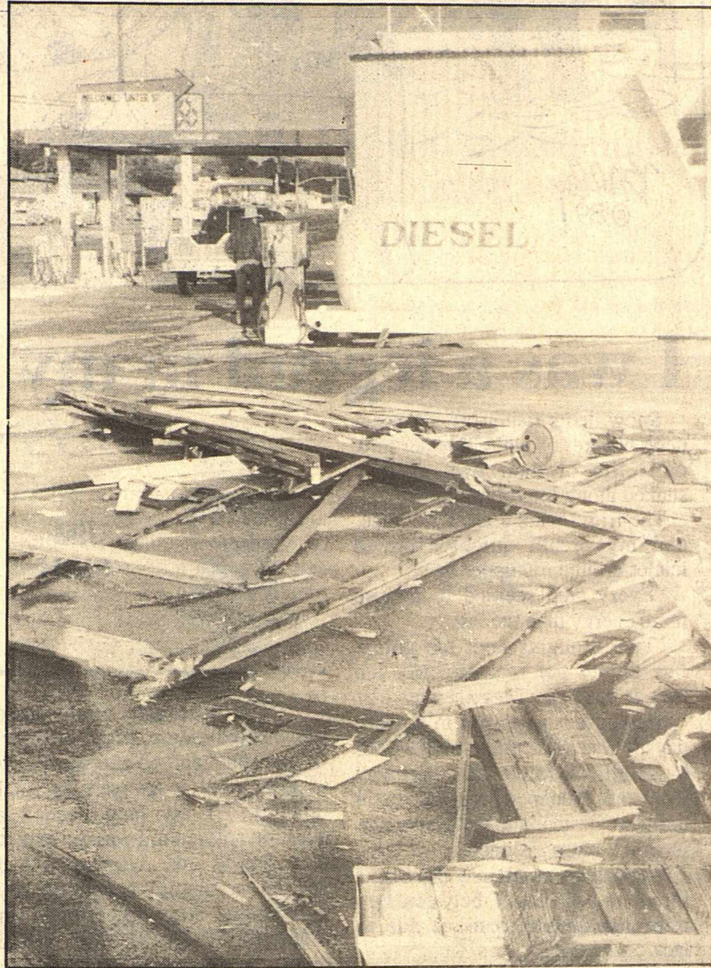
RAISING THE ROOF - The Bait Stop was one of several Sonora buildings damaged by Monday morning's little twister.
