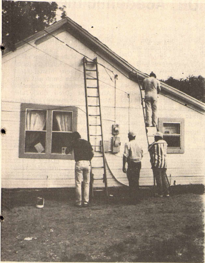
HOME SWEAT HOME - Sonora volunteers break a sweat making needed repairs on this Christmas in April project.
