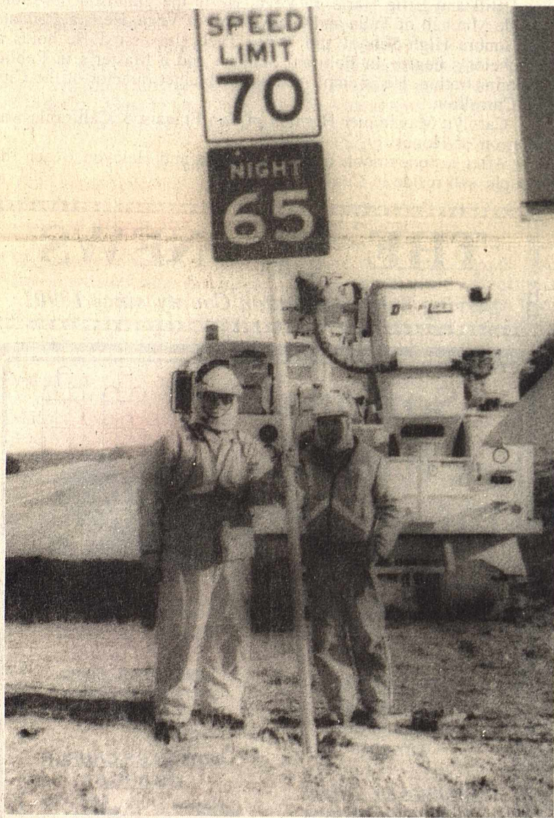
Texas Department of Transportation employees, Ronald Lee Morgan and Joe Sherman, place a 70 mph speed limit sign on Highway 277 North to San Angelo.
