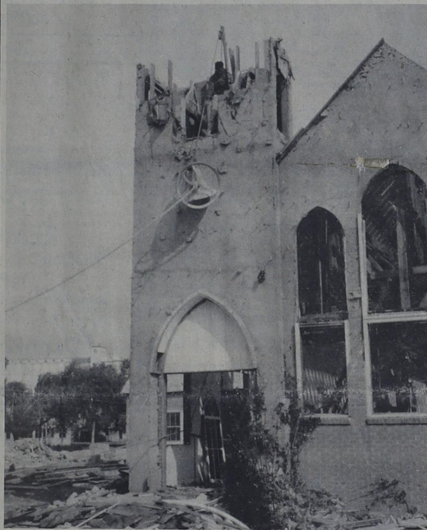
COMING DOWN -- After being taken loose from its position in the tower, the bell is being lowered to the ground. The rope in left foreground was attached to Dorsey's pickup. Members of the Methodist Church hope to make use of the bell in the future.
