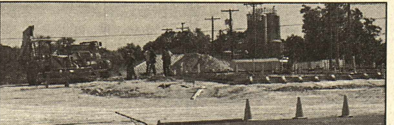
This construction taking place next to Skinny's convenience store on 277 N. may have caught your eye and left you wondering what was coming to town. For those that don't know yet, it is to be a Best Western Motel and R.V. parking.
