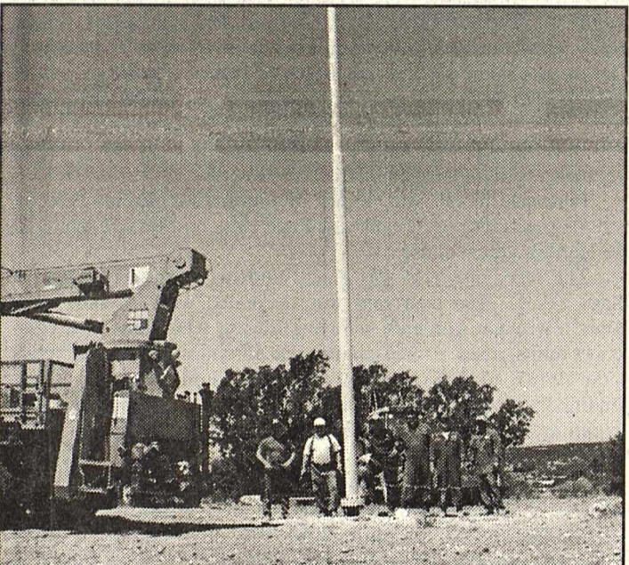
Workers from Schlumberger and the Sonora Industrial Development Corporation worked together on Friday, May 31st to set the 60 foot flag pole on top of Eaton Hill. The flag will be raised in a special ceremony on Tuesday, June 11, 2002 at 9:30 a.m. A very special thank you goes to Jimmy Cahill and Cahill Construction for all that they have done to make this project possible.
