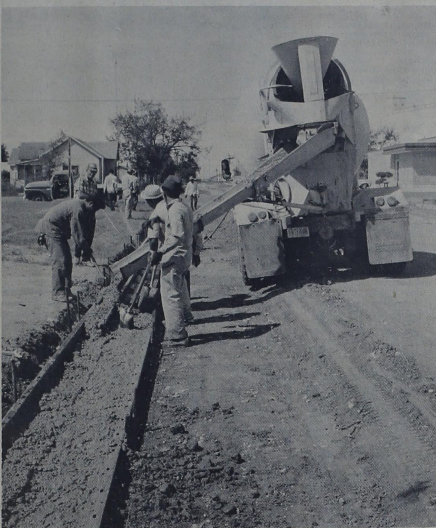
STREET IMPROVEMENTS -- Curbs and gutters were being poured last week and this on several blocks in Bovina which are included in the current paving program. This crew is distributing cement in forms for curbs and gutters on Avenue A between Second and Third Streets. Curbs and gutters were installed on seven blocks last week.
