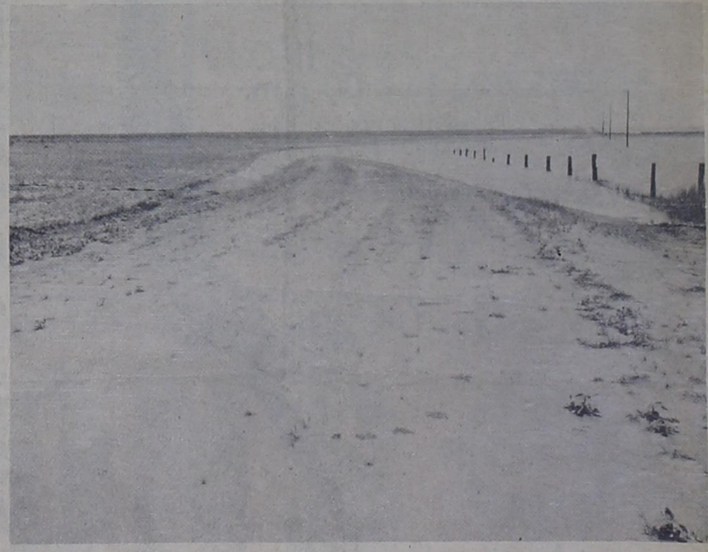
LAKE ROAD ---- Offering proof that there has been more rainfall than usual in the area this year is this water-filled county, all-weather(?) road located a mile east of FM Road 1731 three miles south of Bovina. The road is considered a permanent one and hadn't been overrun by the lake at right for any length of time in years. Rains during the past few weeks, however, have crowded the lake out of its banks and made the road unusable. This view is looking south.
