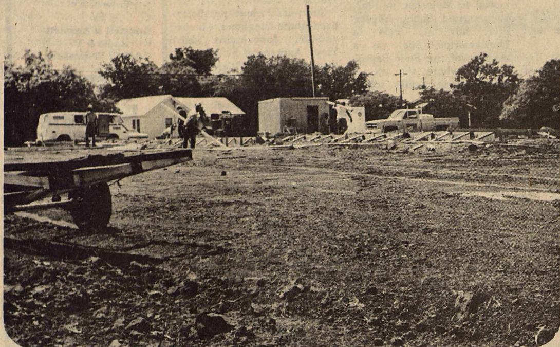
CONSTRUCTION ON 28 Units of rental housing in Haskell is underway. The housing will be located on South 277 and S. 6th streets. Cost of the project is approximately $460,000 and should be completed in about six months. (Staff Photo)
