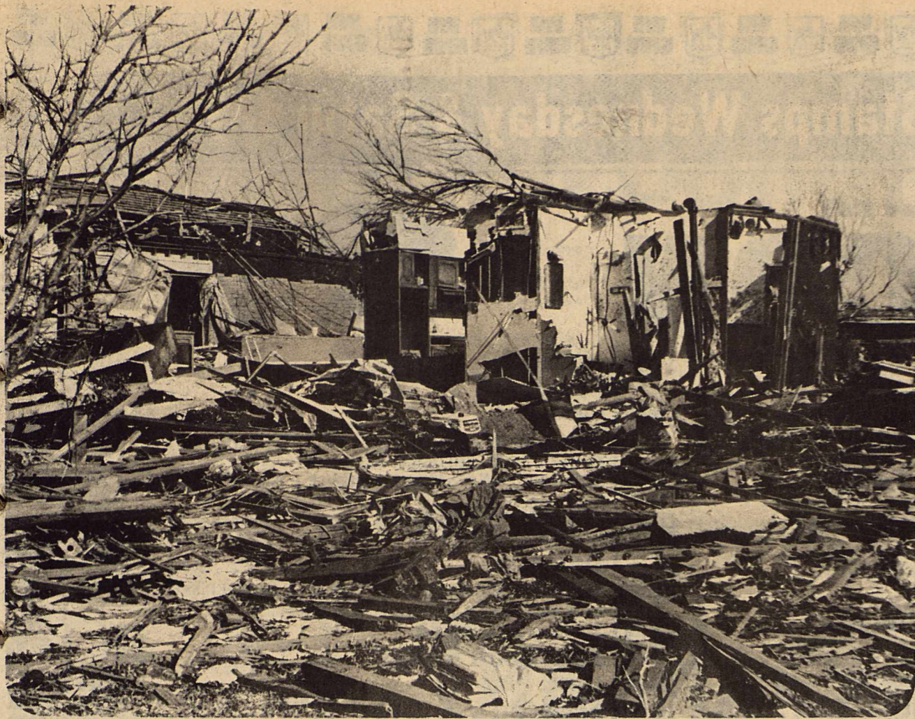
WICHITA FALLS DAMAGE... Homes in the path of a killer tornado in Wichita Falls April 10 were completely destroyed. Many Haskell residents have expressed a desire to aid victims of the storm and Wichita Falls
