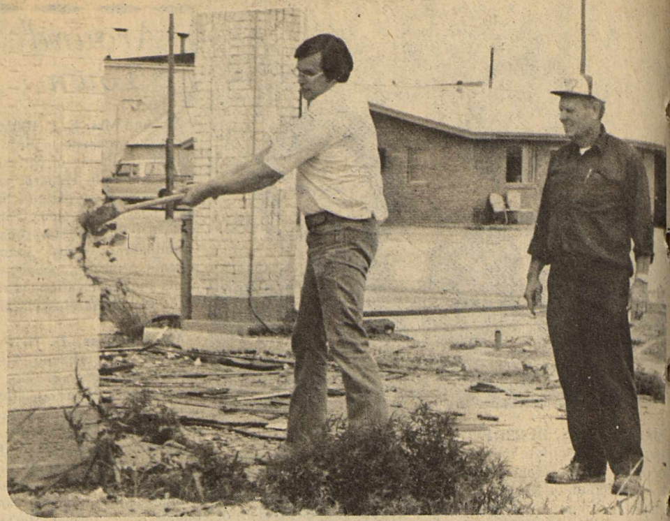
DESTRUCT AND START OVER... Jimmy Bynum and John Larned recently began removal of a vacant gas station at 2nd and U.S. 277. Following the removal of the station, the two plan to build a motel and
