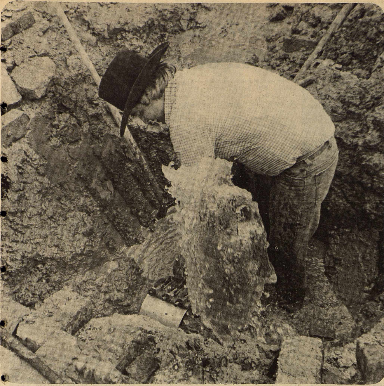
ALMOST UNDER CONTROL...A water leak in an eight inch main on the south side of the square Monday resulted in turning off water to all city customers for
