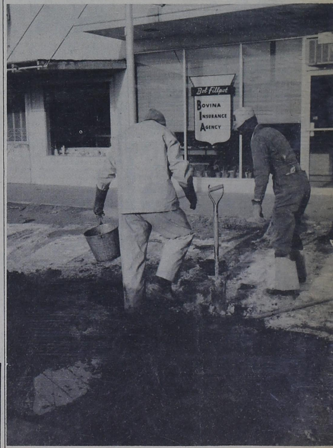
COLD WEATHER WORK --- Darrel Read, left, and Leon Clemons, city employees, search for a broken water line under frozen Main Street in near zero temperatures Tuesday morning. Read says the origin of the leak was undetermined but figures the cold weather was involved, directly or indirectly.
