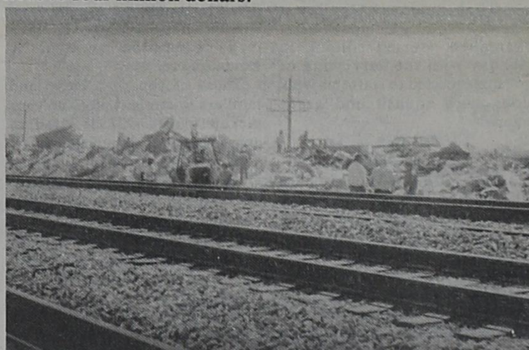
CLEANUP CONTINUES...The cleanup continued this week at the Santa Fe Railway derailment site. The repaired track is shown in the foreground, as traffic has been restored to its former level.
