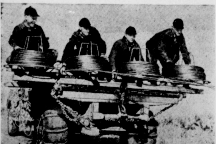
Stringing four lines of aluminum cable at once near Horton, Kan. REA projects have required 115,000 miles of this cable.
