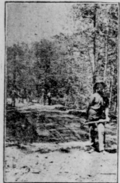
GETTING THE GRADE READY FOR STONE. (From Good Roads Magazine, New York.)
