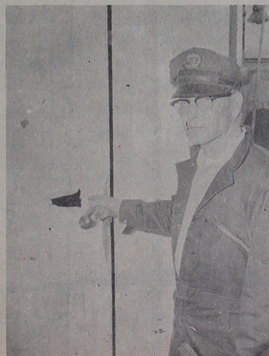
ENTRANCE--W.H. Rogers of Bonds Oil Co. points to a hole in a rear door of the station building which burglars made Sunday night to gain entrance to the building. Approximately $900 was stolen in cash, checks, and credit cards.
