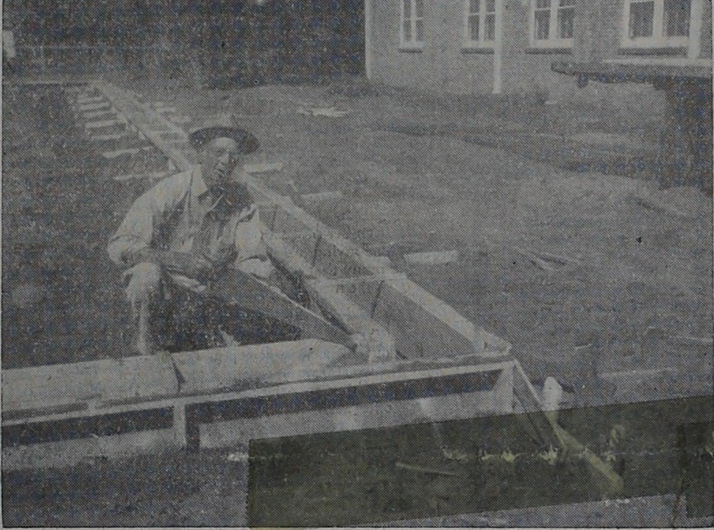
METHODIST CONSTRUCTION BEGINS — Work began last week on a new educational building for Bovina Methodist Church. The building, to be 43 by 96 feet in size is being built just north of the present building. The north side of the church may be seen in the upper right corner of the picture. Hubert Ellison, pictured, is in charge of construction.
