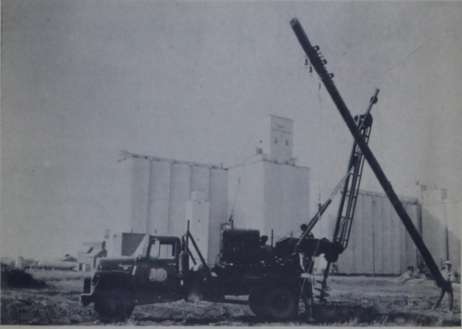
TIMBER-R-R-R! —Southwestern Public Service Co. workmen unearth a power pole with a drill-and-hoist rig to clear the construction site for Dimmitt Wheat Growers' corn milling plant complex in East Dimmitt. SWPS crews have removed 20 or more poles at and around the plant site. Con-
