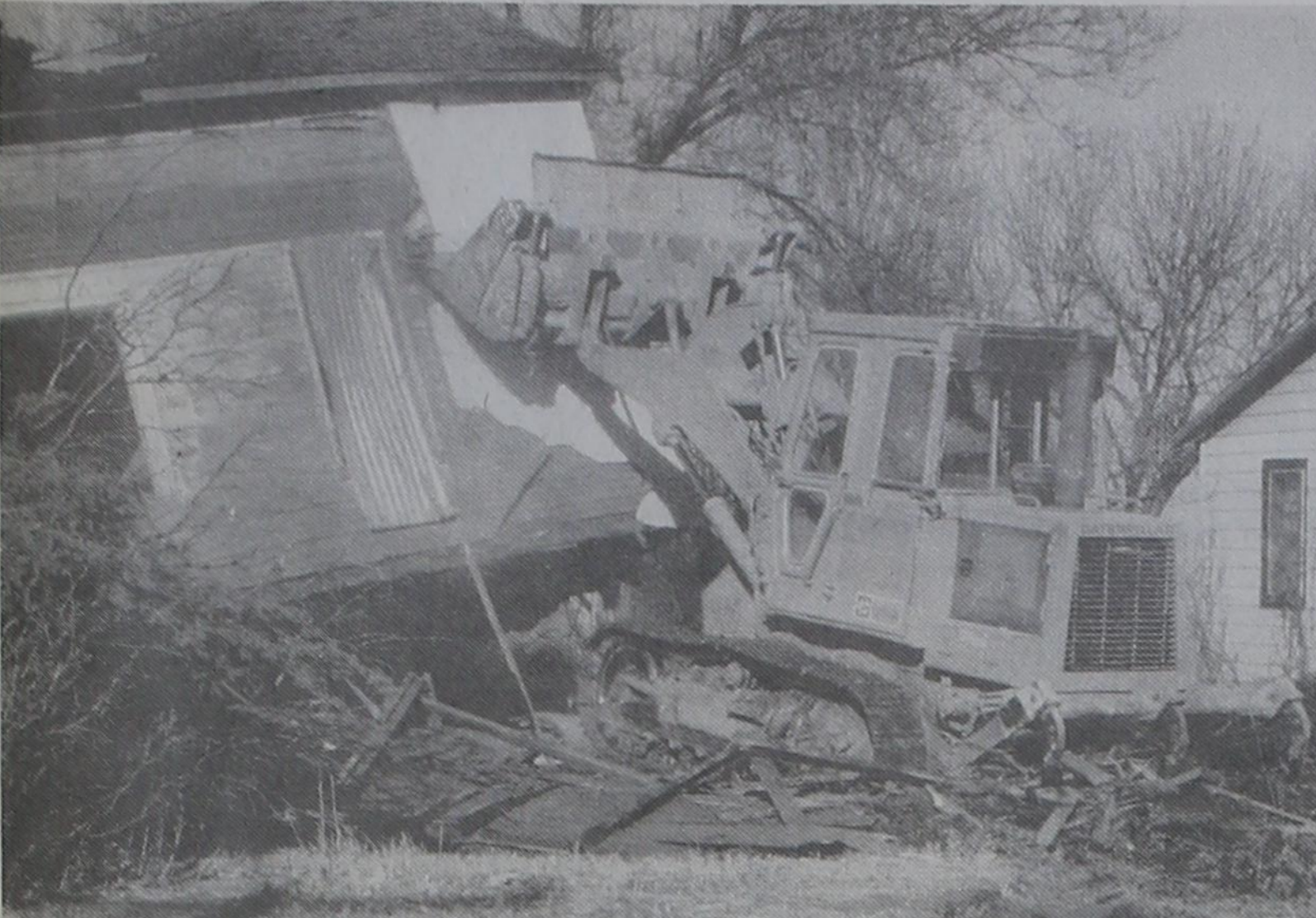
UPSY DAISY — This house at 407 Northwest Eighth Street in Dimmitt is being demolished Tuesday morning by a city bulldozer operated by C.C. Lopez in response to neighbor complaints
